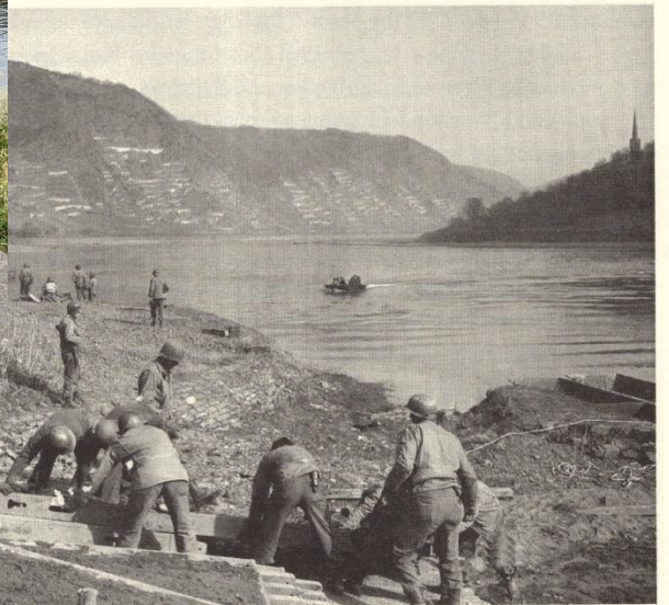
Koblenz, Germany—16 March 1945. Engineers begin construction of a bridge across the Moselle River at the site of the 347th Regiment's crossing.
